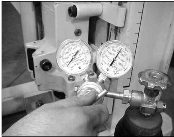
Figure 7. Adjust fill line pressure to 350 psig.
